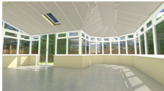
3 layers of high performance insulation (between and over rafters, and insulated plasterboard), is installed.
