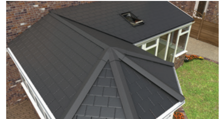
Chosen tile is added ensuring weathertightness and the gutter and external trim are secured in place.
